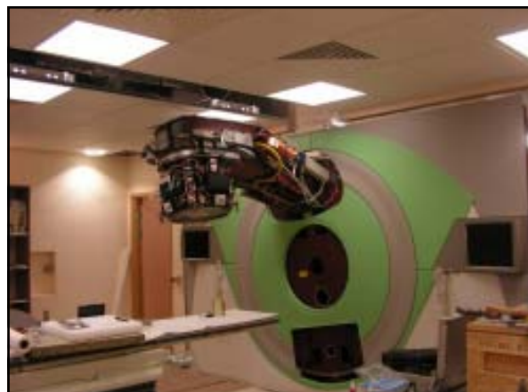
The first linear accelerator being installed
