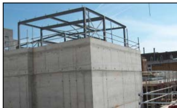
Completed Linac walls and roof slab, with first floor steel frame in place
